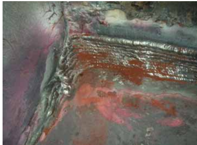
Final repair weld on the inside between the AFT wall plate and the inner bottom plate of the sea chest at frame 52.
