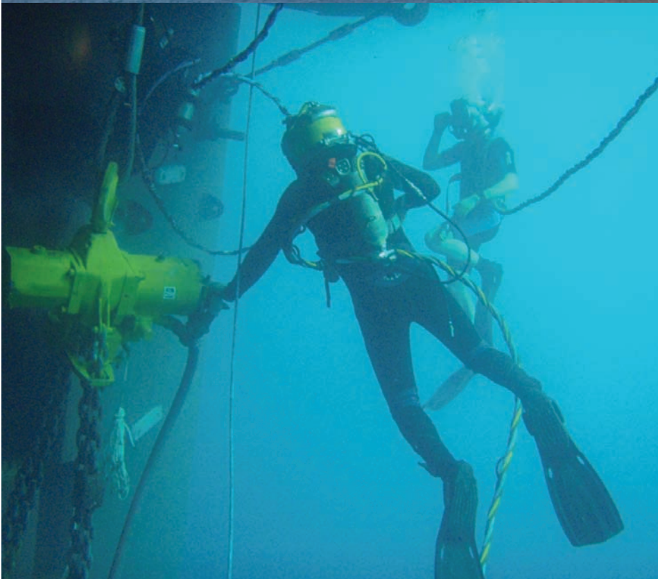
Fig. 2 — Diver operating a 25-ton air chain hoist during removal of the rudder.
